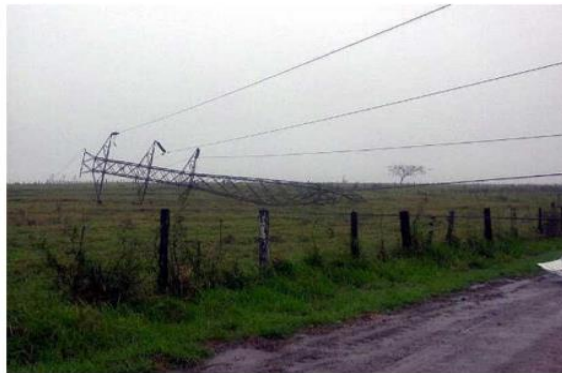
Figura 26 – Torre Colapsada, Sumaré – SP (2012)
